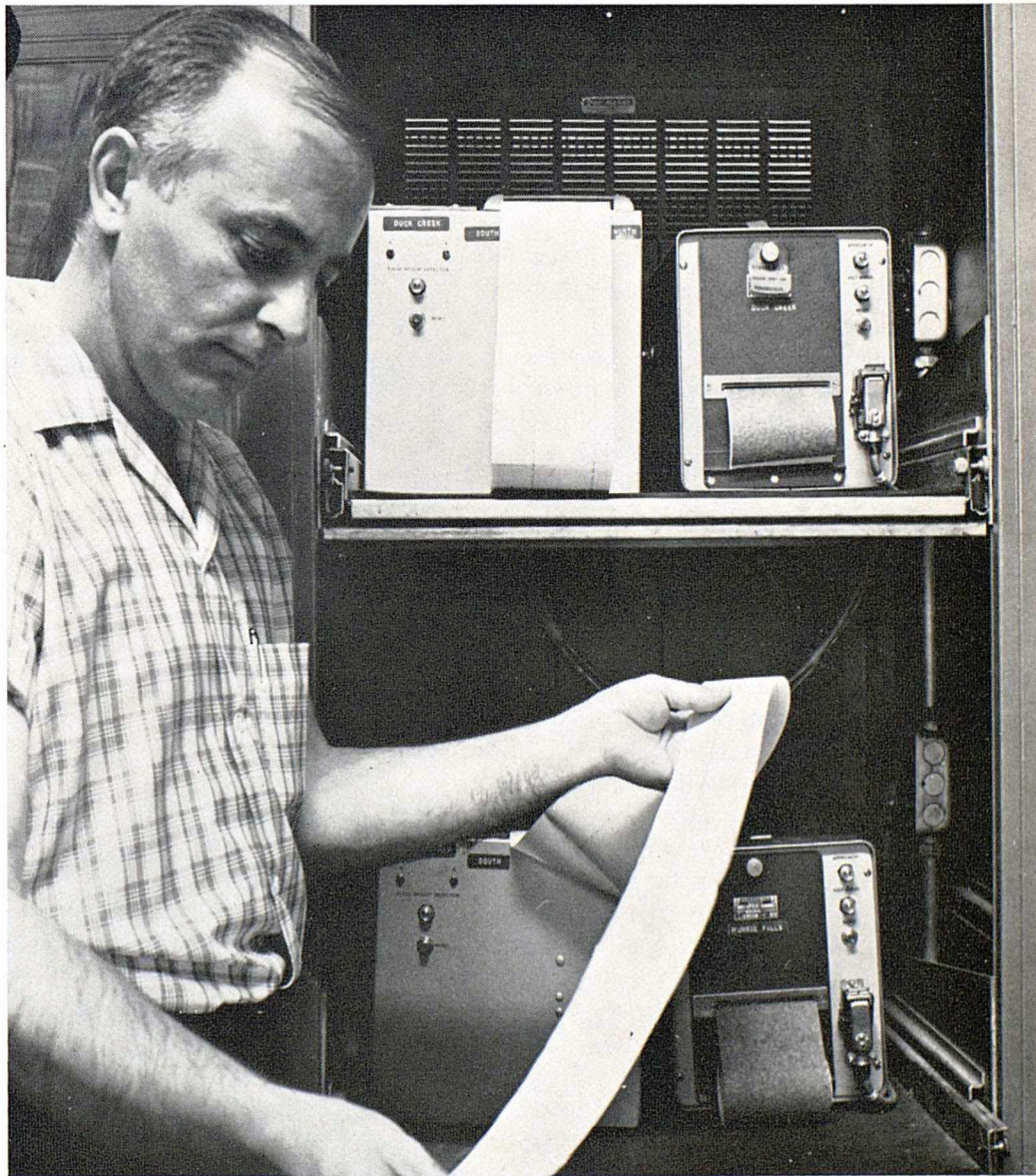
Recorders (left) and wheel counters (right) are in the dispatcher's office at Akron, Ohio. Readout includes train direction, time of day, and journal data.
